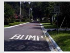
Pavement marking legend "BUMP"
